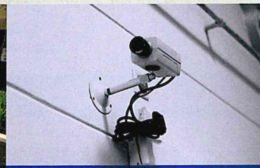
CCTV at Guard House
